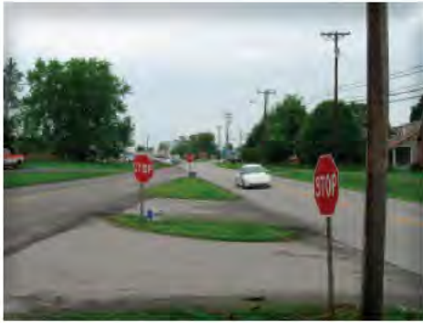
Merger of South Columbia Avenue and MLK Jr. Blvd., showing confusing curb cuts
